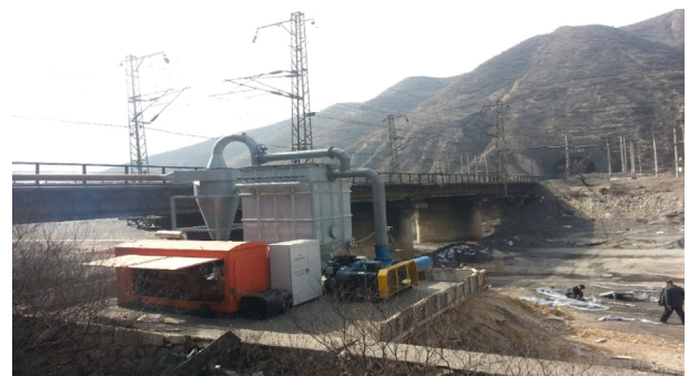
Fig. 5. Coal-dust removal device at the entrance of Zhangjiawan tunnel
