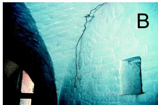
Fig. 4. Characteristic to Heterotermes sp., the thin and nonbranching foraging tubes often hang freely from the wooden beams on the ceiling (A). Although the walls and some floors of the fort are made of brick, termites appeared to tunnel through the mortar joints (B).
